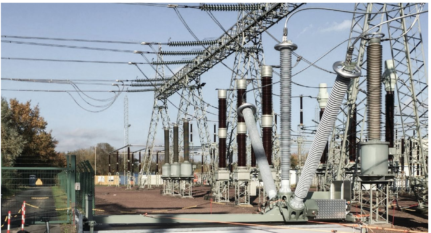
Figure 5: Mobile RC-divider for temporary measurement of power quality in the transmission grid (substation Unterweser)
