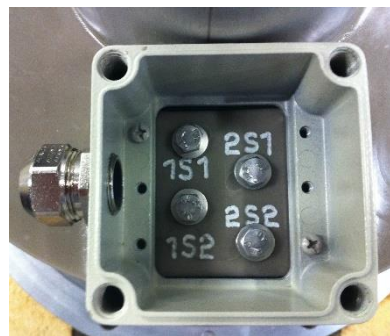
Fig. 8: Example of cable box and nameplate for a current transformer with two cores
