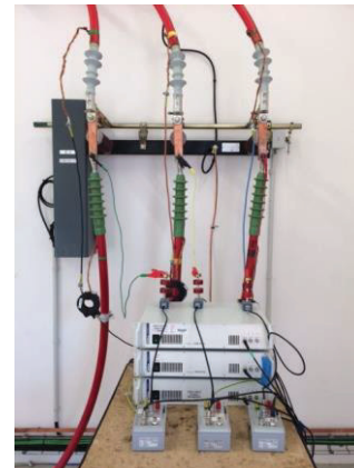
Fig.8. Measuring setup installed on 3-phases.
