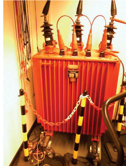
Figure 7: Distribution transformer (HV = 10.5 kV, LV = 400 V).
