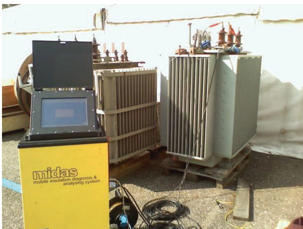
Figure 10: Distribution transformers from Brown Boveri (left) and Breda (right).
