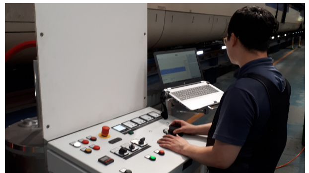
Step 4: After a retrofit with exchange of termination on the train, we recommend to perform a partial discharge test of the retrofit cable with EGT-75 to guarantee the quality of the assemble process.
