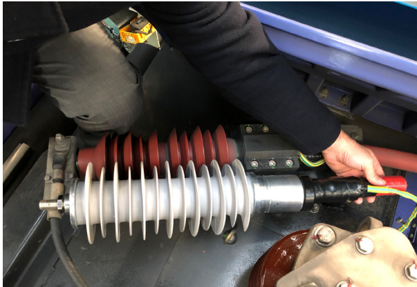
Step 1: Analysis of the installed components, on site on the train or at ALPHA. Examination of the interchangeability of components.
